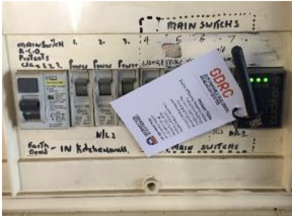
Figure 3. Example installed WattWatchers Auditor 6M
